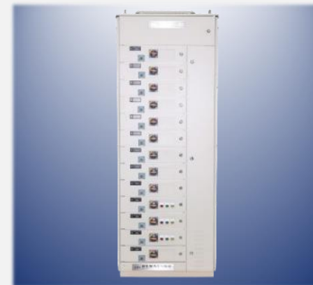
Motor control center (MCC-Xcell Type, IEC- 61439-2)
